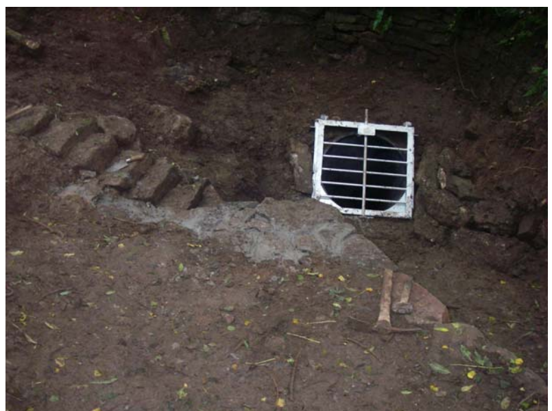
Longwood Valley Sink debris grill and gate. Photo G.J. Mullan
